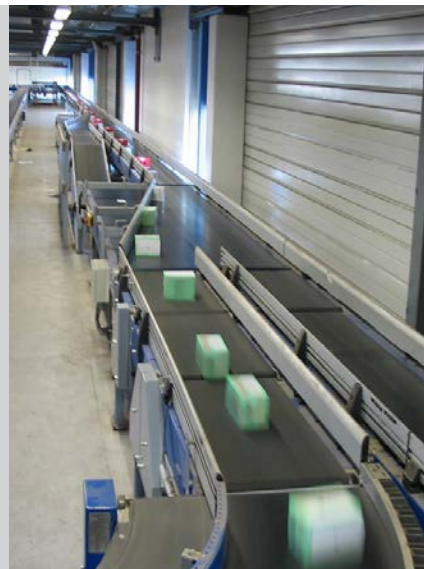
Circulating conveyor belt provides a safe transport
